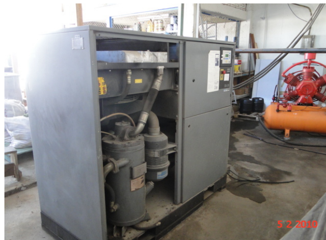
ITEM 108 – COMPRESSOR ATLAS COPCO
